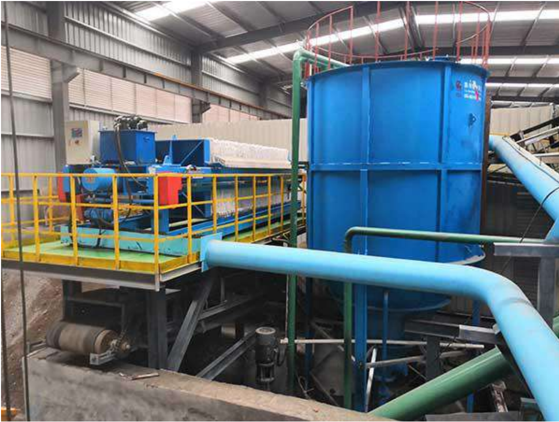
Sludge dewatering for washing plant in Georgia
